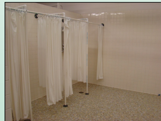
Image 2: Indoor shower facility for decontamination
